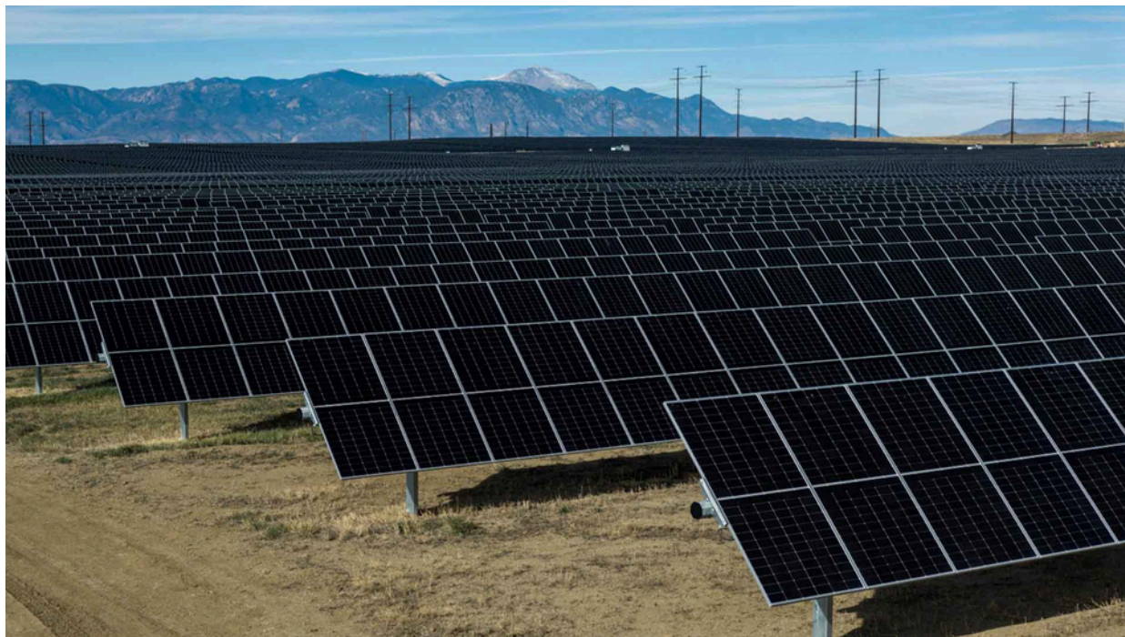
Figure 7: Image courtesy of Colorado Springs Utilities .
